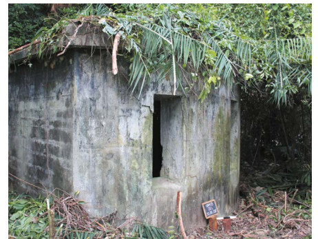
FIG. 4: ONE OF THE DEL EMPLACEMENTS FEATURING STEEL REINFORCED SHUTTERED CONCRETE CONSTRUCTION TO PROTECT THE SEARCHLIGHT EQUIPMENT AND CREW. (CREDIT: AARON KAO)
