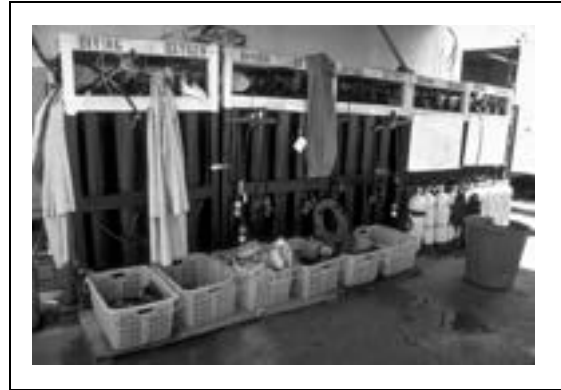
Oxygen racks for surface decompression.
