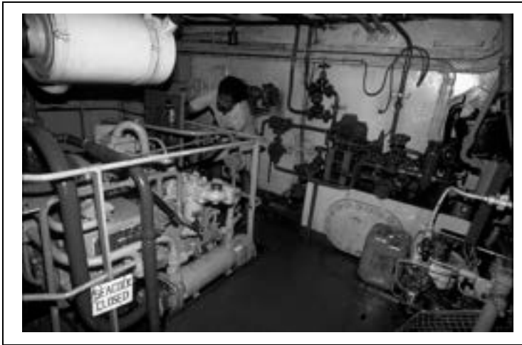
Engine room of ATSA I.
