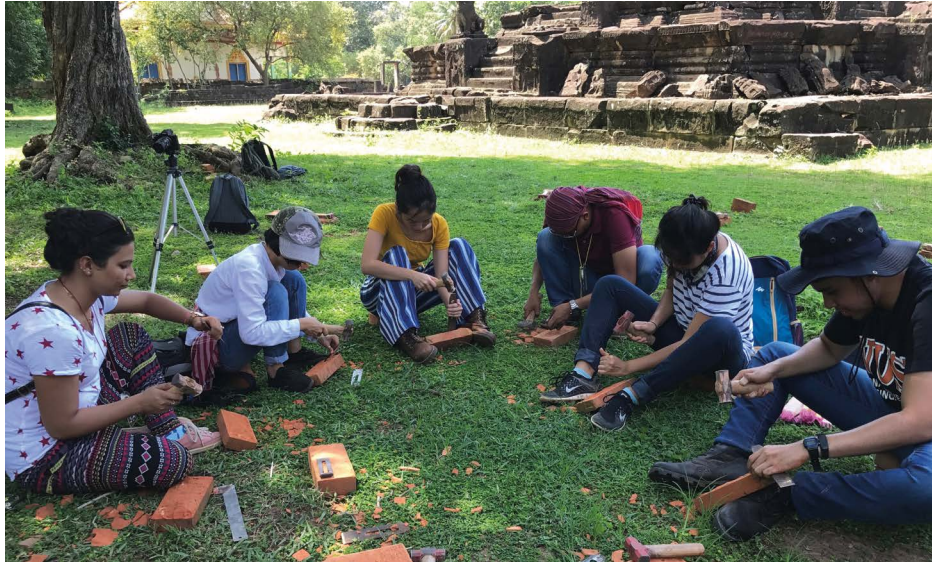
Brick conservation workshop at the 9th century Bakong temple. (Credit: Chan Wai Peng)
