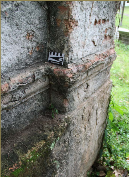
THE MOULDING, PROFILE, CORNICE AND STUCCO/LIME COATING ARE IN GOOD CONDITION FOR FUTURE CONSERVATION WORK. (CREDIT: HÉLÈNE NJOTO)
