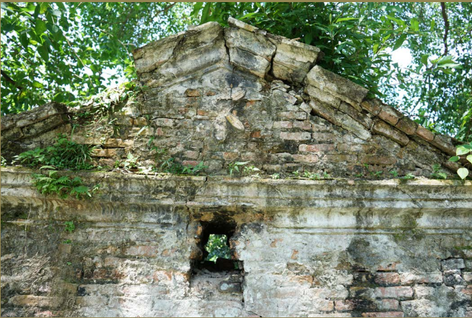
WESTERN FAÇADE OF THE BUKIT KASITA GATE (REAR FACADE), LIME COATING REMAINS AND MASONRY WORK. (CREDIT: HÉLÈNE NJOTO)
