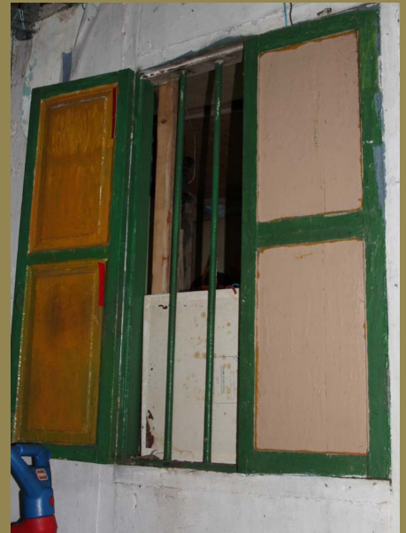
ONE OF THE ORIGINAL WINDOW FRAMES AND SHUTTERS (SOUTHERN WALL). (CREDIT: HÉLÈNE NJOTO)
